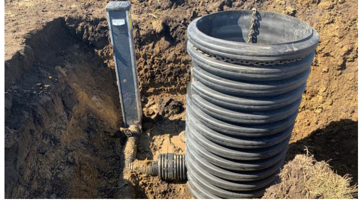
Figure 3. Gate Structures to Control Water Table
