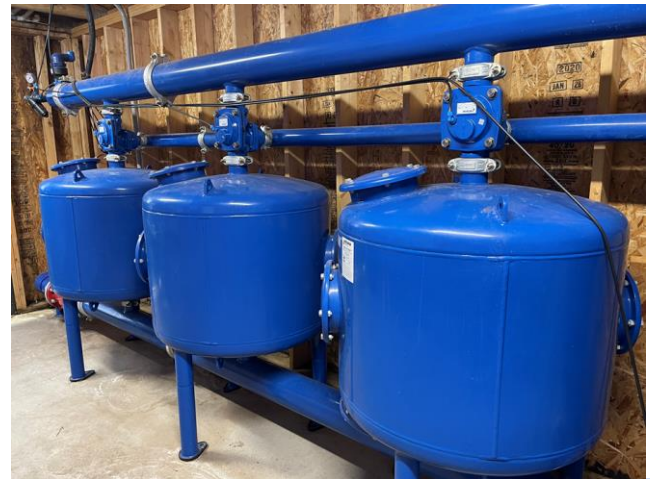
Figure 9. 3-Stage Sand Filtration System
